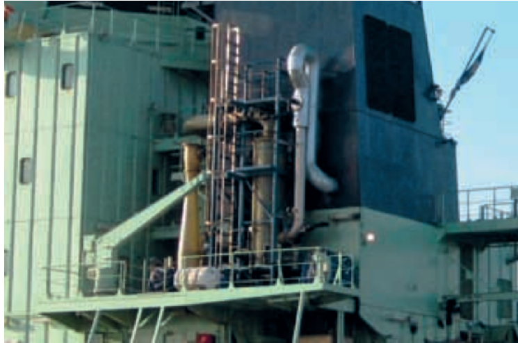
Figure 21: External exhaust gas scrubber
