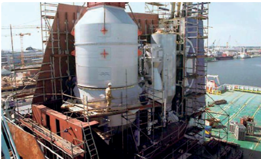
Figure 22(a): Alfa Laval scrubber installation on DFDS ro-ro
